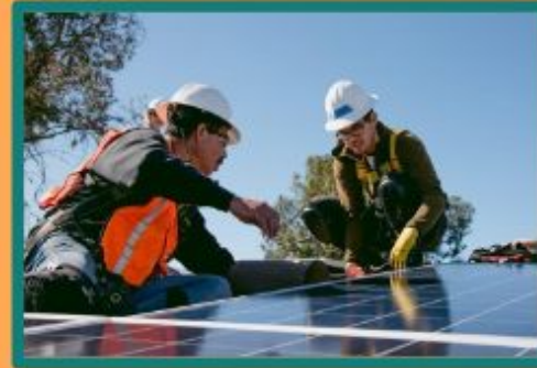
Oscar, a SOMAH job trainee, supports the solar installation at Loma Sierra Apartments.
