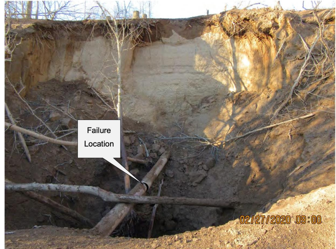
Figure 6. Failure Location (Upstream to Downstream)
