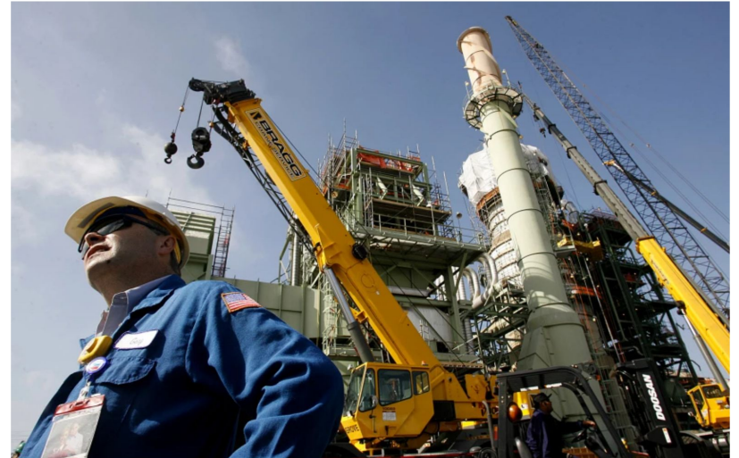
Chevron oil refinery manager Gary Yesavage stands next to a major piece of equipment that is being overhauled in El Segundo, Calif., on June 14, 2007. (Wally Skalj / Los Angeles Times)
